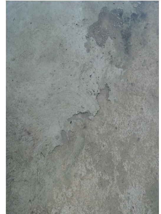
Slab before Repair
